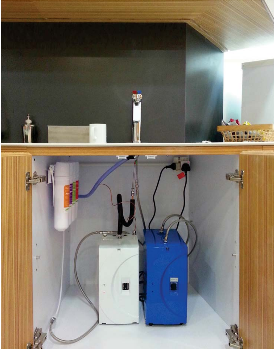
Undersink "Boiler & Chiller"
